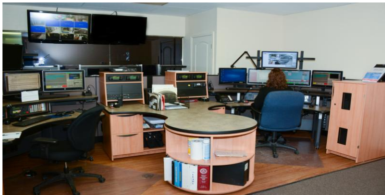
Safety Communications Center
